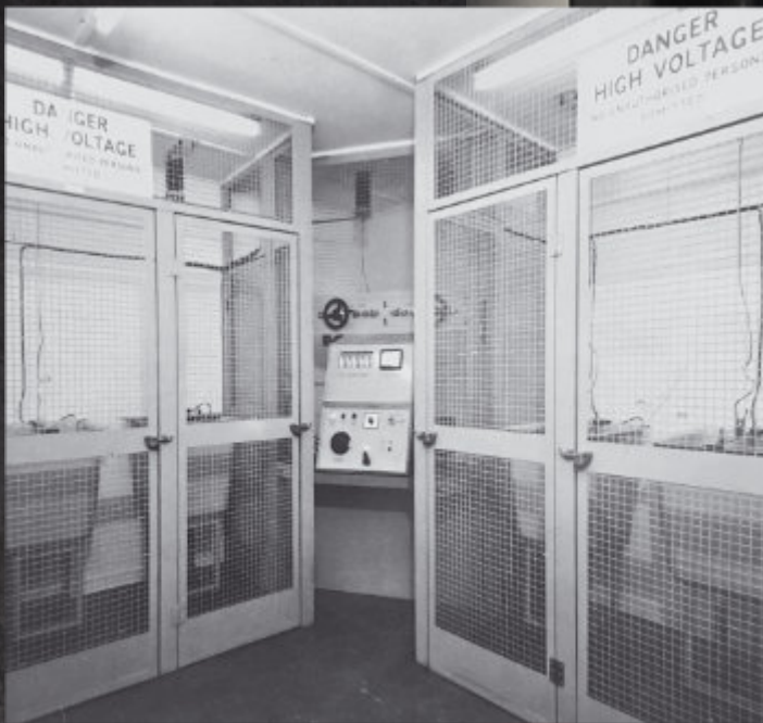
Our electrical testing facility circa 1983
